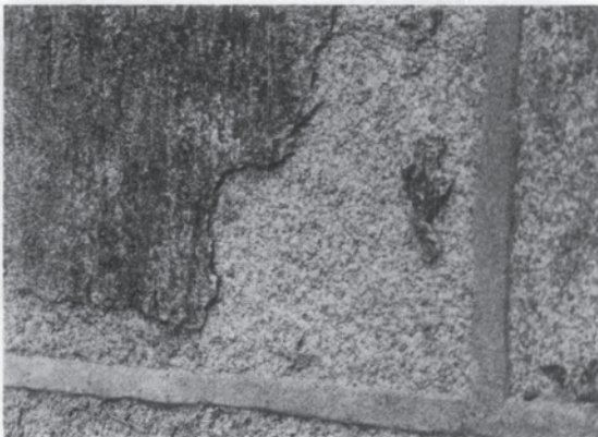
Peeling of granite. Photograph: Baird M. Smith, AIA.
