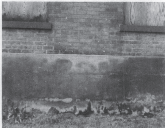
Rising damp evidenced on parged foundation. Photograph: John Stubbs.
