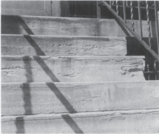
Differential erosion of sandstone steps follows bedding planes of greater and lesser resistance. Photograph: Anne E. Grimmer.
