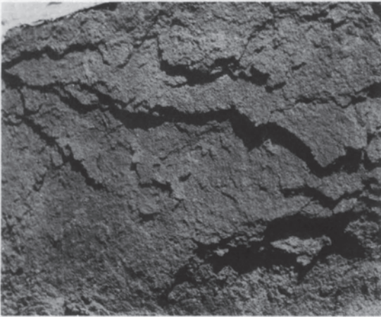
Exfoliation of sandstone. Photograph: Anne E. Grimmer.
