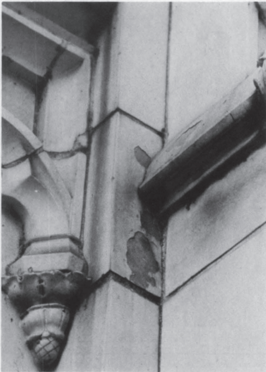
Glaze spalling of glazed terra cotta. Photograph: John H. Myers.
