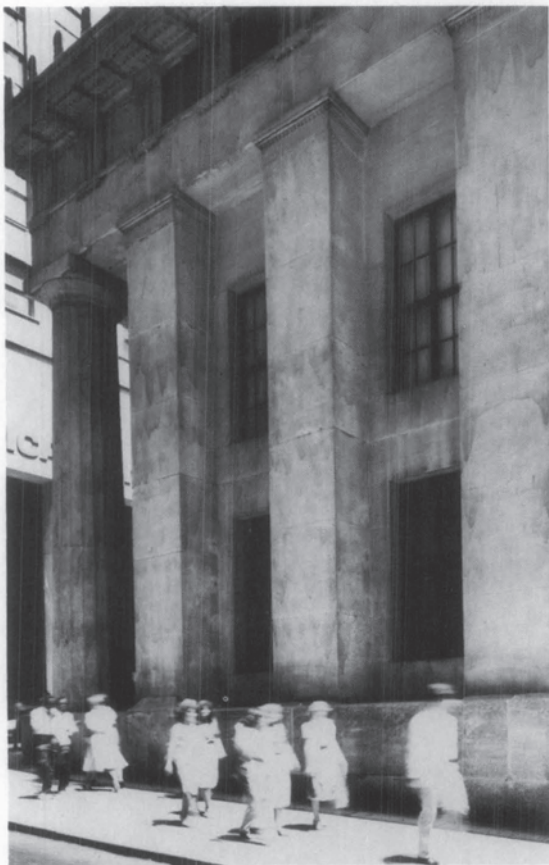
Water-repellent coating improperly applied gives a blotchy appearance to the stonework. Photograph: Walter Smalling.
