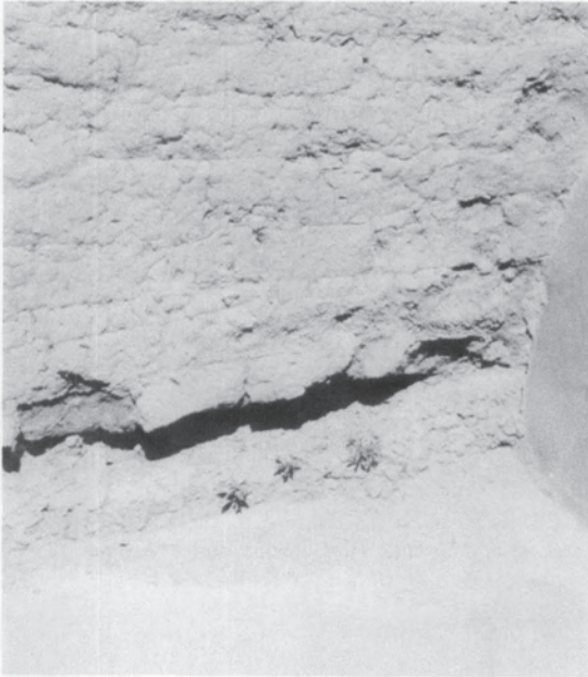
Coving of adobe wall. Photograph: National Park Service.
