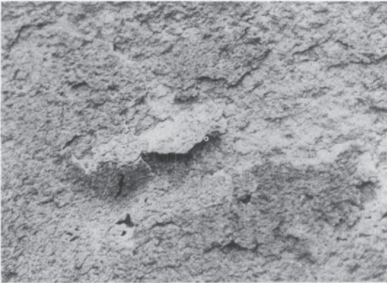
Flaking of granite. Photograph: Baird M. Smith, AIA.
