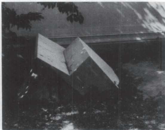
Section of marble lying on the ground at base of building after it had separated from pediment above. Photograph: Walter Smalling.
