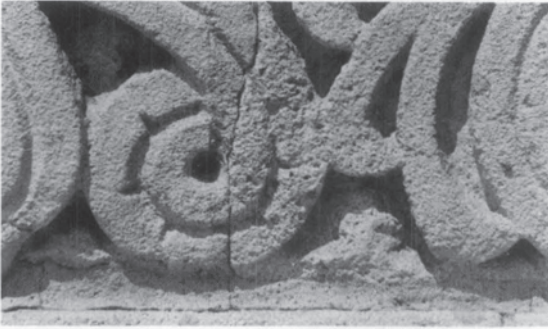
Cracking of limestone. Photograph: John H. Myers.
