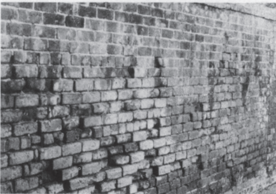
Efflorescence and spalling on brick wall. Photograph: Anne E. Grimmer.
