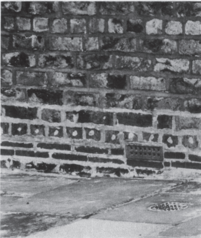
The horizontal row of white dots in the brick headers indicates that a chemical dampproof course has been injected. Photograph: Baird M. Smith, AIA.
