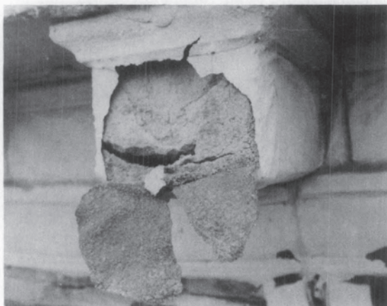
A neoprene coating over a limestone cornice has trapped water (which entered through leaks in the parapet) inside these stone dentils. The built-up water pressure has finally forced the coating to pop off, taking with it pieces of the stone. Photograph: National Park Service.
