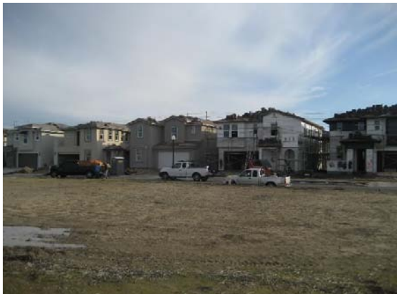
Looking south across Tax Zone 6 lots (Lennar) at homes under construction by Anthem United in Tax Zone 7
