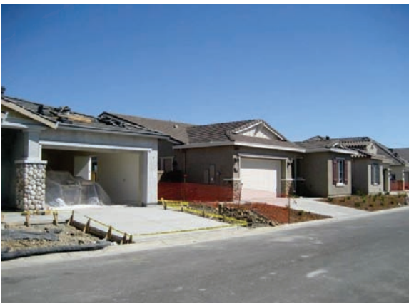
Homes under construction in Village G/C (K. Hovnanian) (Photo Taken on September 18, 2016)
