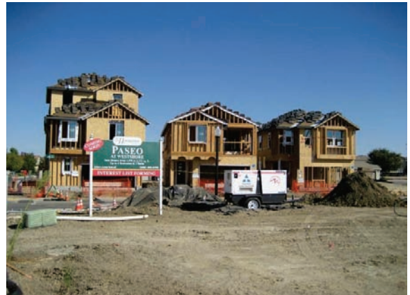
Models under construction within Village F (K. Hovnanian) (Photo Taken on September 18, 2016)
