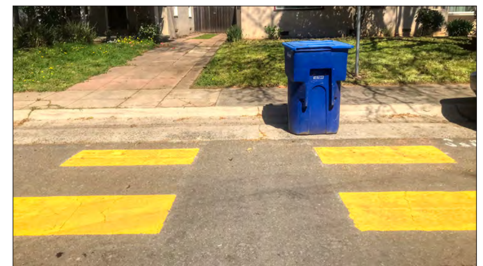
The existing crosswalk at 7th Avenue and Cutter Way lacks ADA-accessible curb ramps.
