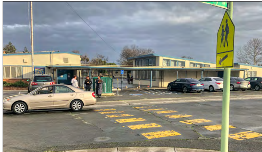
Crosswalk marking across Strawberry Lane at 27th Street is worn and should be refreshed.
