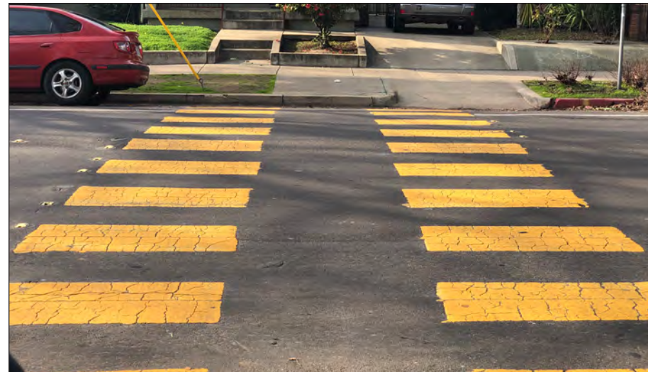
The east leg of the crosswalk at Alhambra Boulevard and I Street lacks an ADA-standard curb ramp and terminates at a residential driveway.
