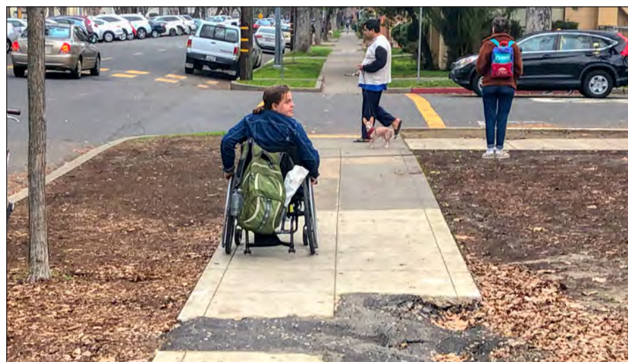
The broken concrete sidewalk on 8th Street presents an accessibility issue..
