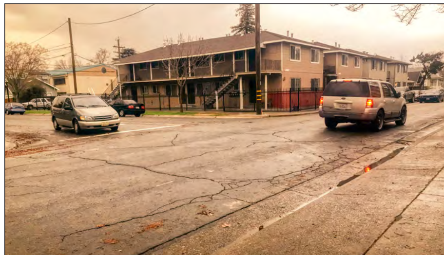
Offset driveway at the intersection of Y Street and 36th Street requires awkward vehicular movements and confusing routing for pedestrians crossing the street.
