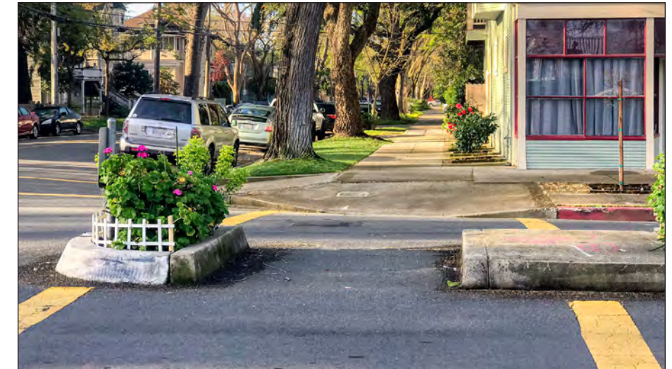
Several curb ramps in the vicinity of the school are missing a detectable surface treatment, i.e., truncated domes.
