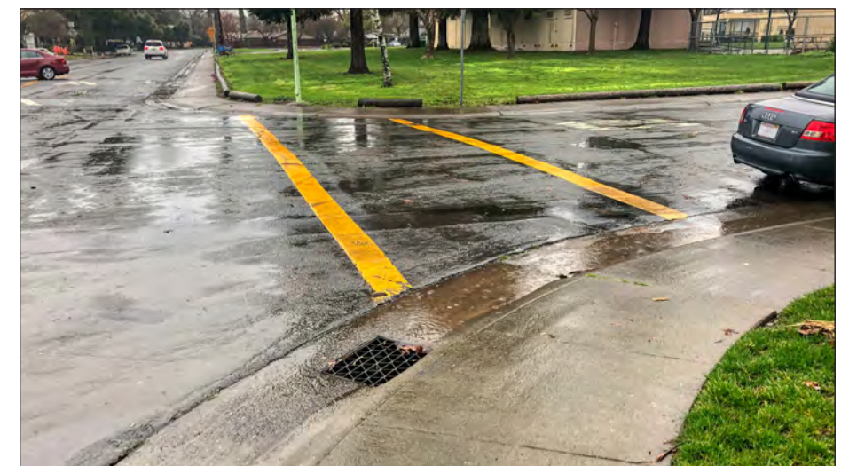
Many crosswalks near the two schools lack ADA-compliant curb ramps (shown: Grandstaff Dr and Bamford Dr)
