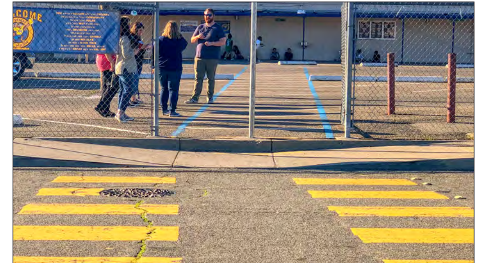
The transition between the internal walkway and the sidewalk along Larchwood Drive is separated by a raised curb, resulting in a non-ADA compliant route.
