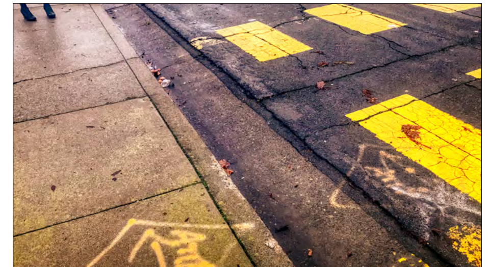
Several crosswalks along Y Street lack curb ramps.
