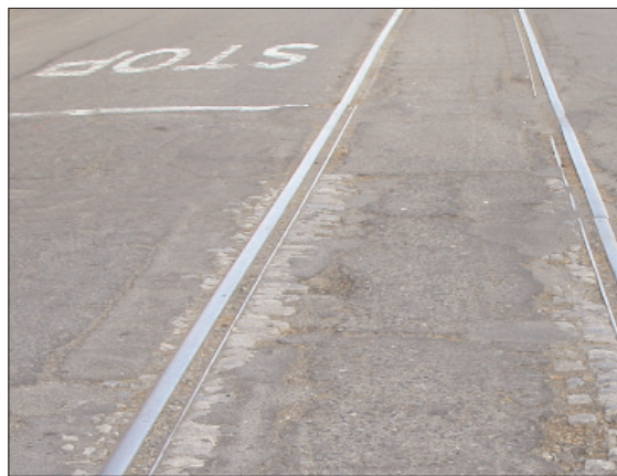
Abandoned rail tracks on R Street contribute to the varying pavement conditions in the area.
