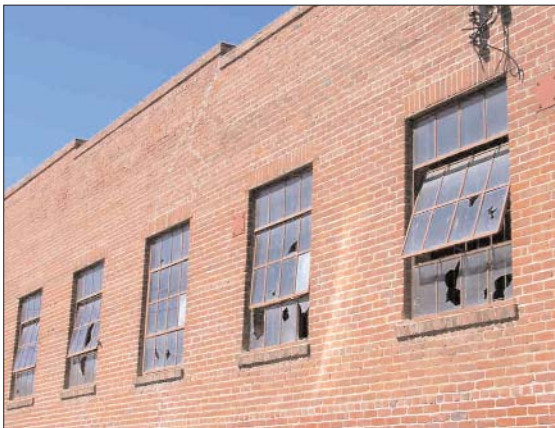
Broken windows fronting R Street
