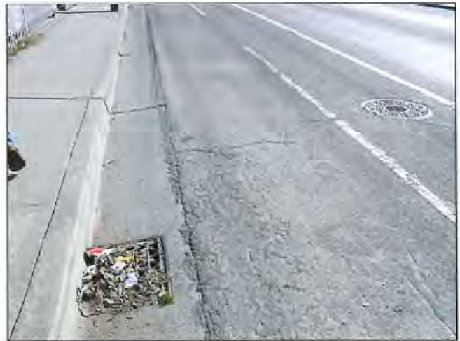
View of existing blocked storm drain inlet
