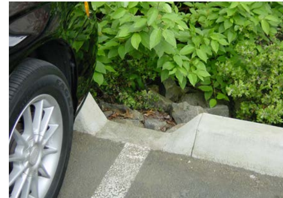
Rain garden gutter detail - Portland, OR
