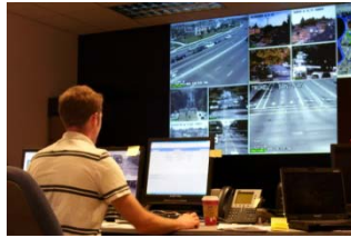
Traffic Operations Center
