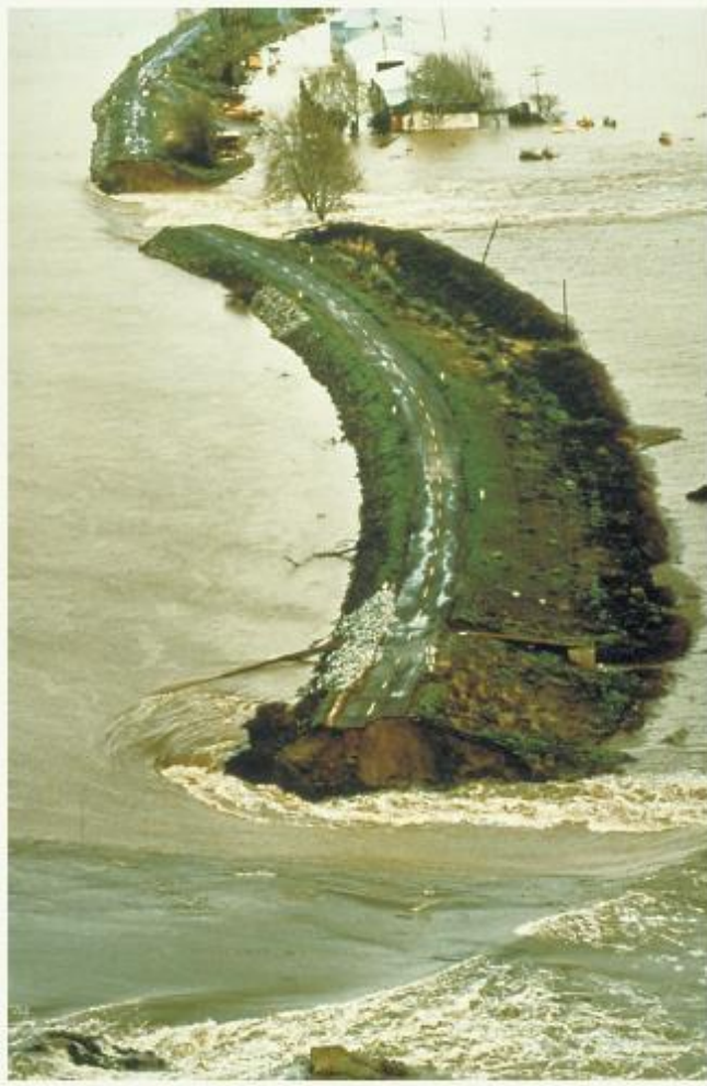
Figure G-10 1986 Tyler Island Levee Breach
