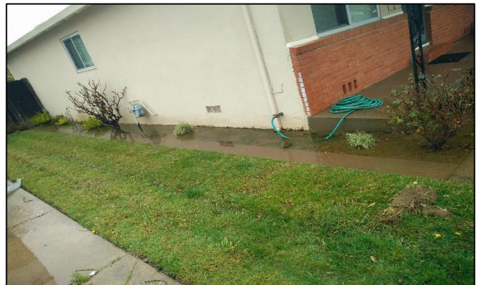
Ponding caused by landscaping obstructions.
