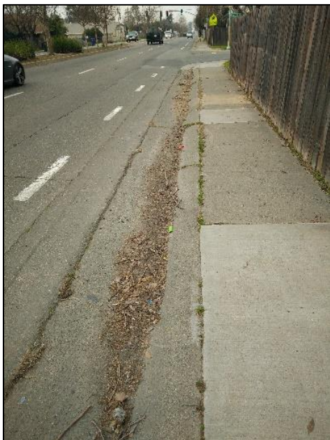
Debris along the sidewalk that can contribute to backed up drains.
