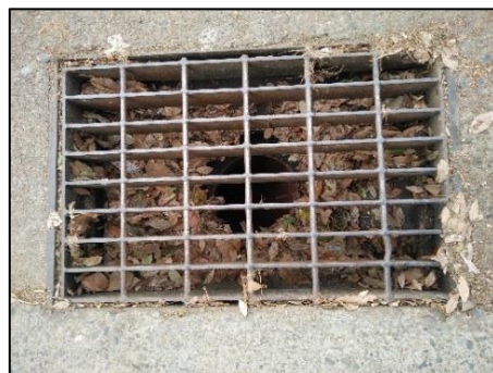
Drains filled with debris as a result of inadequate street cleaning and yard maintenance.
