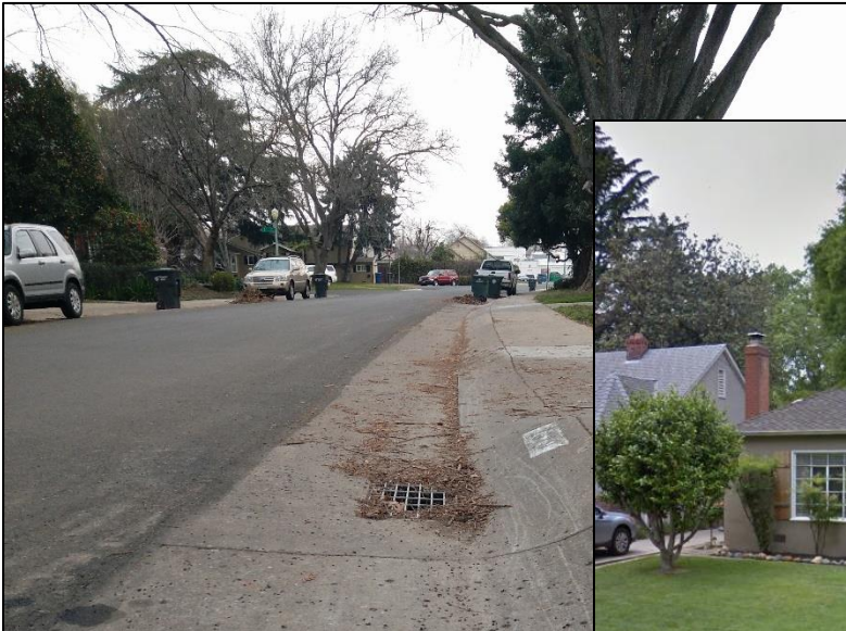
Example of debris in the storm drain. Leaf piles are allowed to be left on streets for City pick up. Many times, these leaves can be sweep down into the storm drain.
