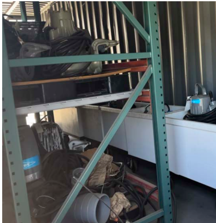
Task A (Photo A6): Inspection of City spare part inventory (view 2) including customized bins and labels for key critical parts such as spare pumps.
