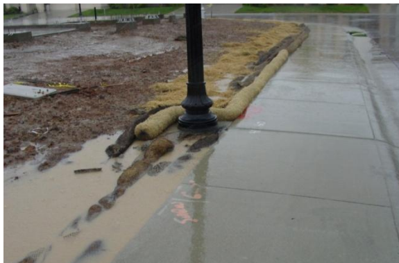
Vehicular traffic will damage fiber rolls and reduce effectiveness.
