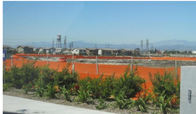
Orange fencing can be used to separate and protect vegetation from construction areas.
