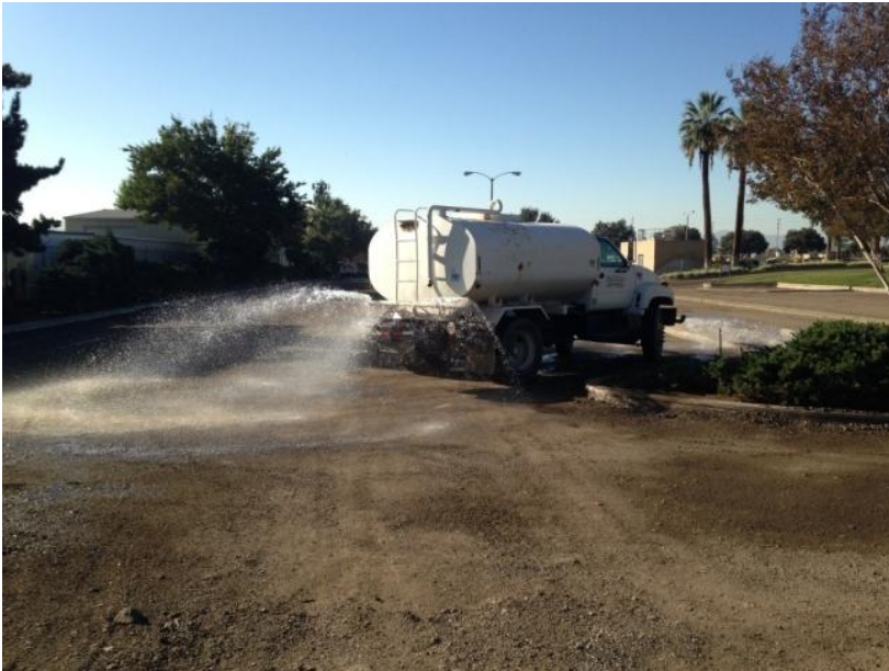
Water trucks can be used to evenly distribute water and avoid causing erosion and/or non-stormwater runoff.
