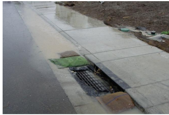
This inlet protection provided limited benefit since sediment-laden runoff is passing easily around the ends of the bags.
