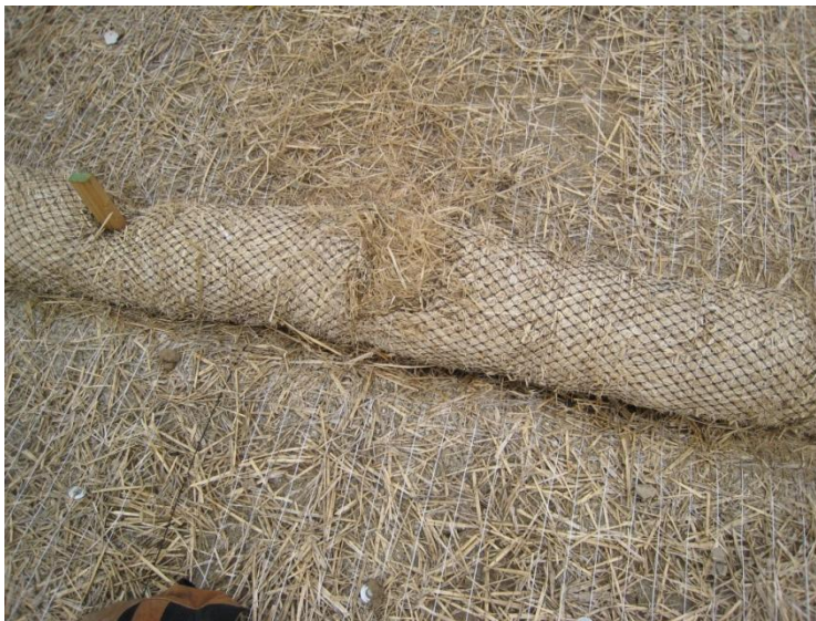
Damaged rolls should be repaired or replaced.
