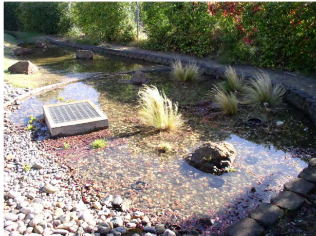
Sand filter in parking lot. City of Sacramento Department of Utilities
