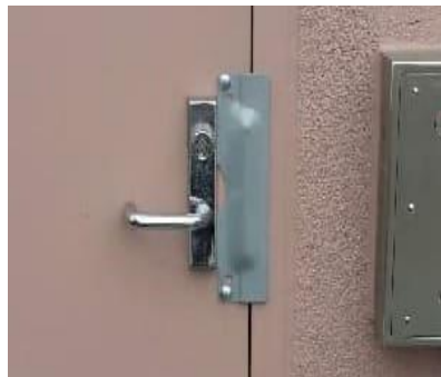
Metal Latch Guard On ALL Out-Opening Exterior Doors
