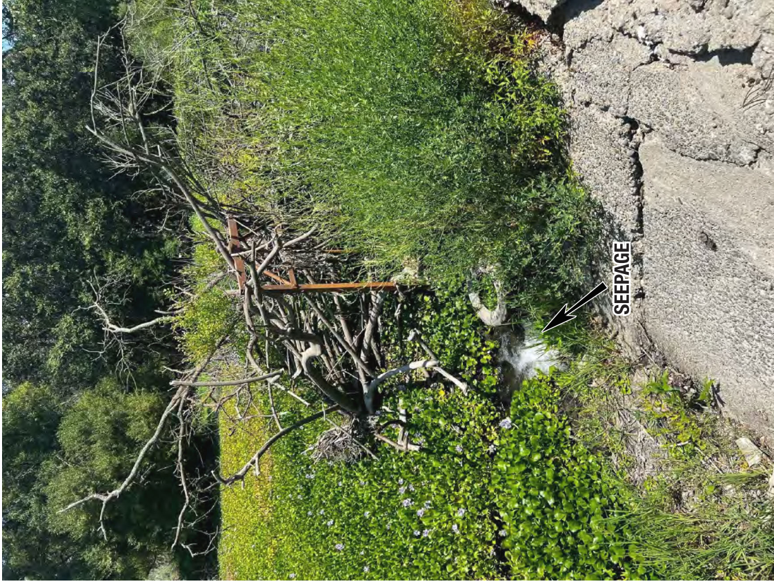
Photo No. 4 Seepage discharge through embankment into Morrison Creek.
