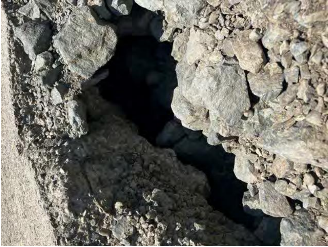
Photo No. 3 Typical Rip-rap/concrete rubble in berm.
