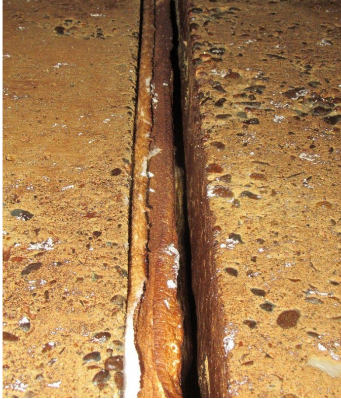
Photo 5 – Expansion joint filler loss/failure
