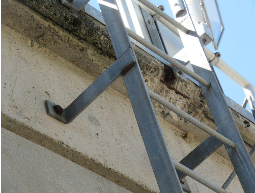
Photo 1 – External reservoir damage impacting structural support for ladder
