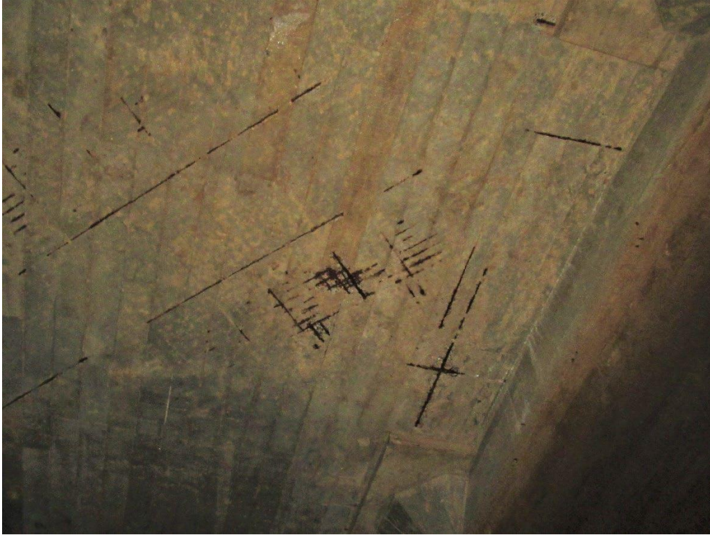
Photo 3 – Ceiling rebar damage within reservoir causing spauling and structural damage
