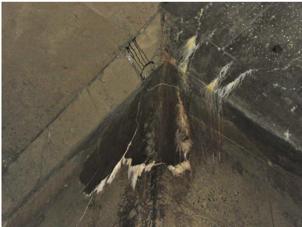
Photo 4 – Reservoir concrete ceiling structural damage from cracking concrete
