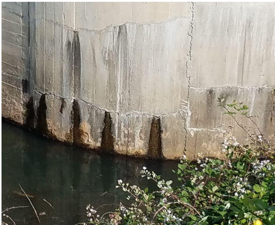
Photo 6 – Cracking damage causing water to leak through
