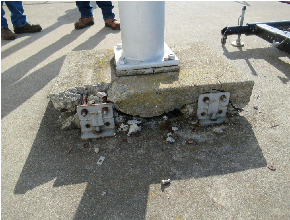
Photo 2 – Structural damage at valve support impacting valve operation
