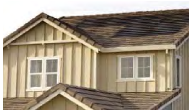
Building integrated photovoltaic panels.
