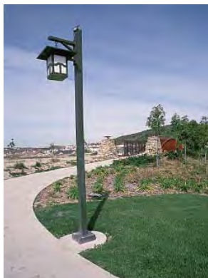
Pole-mounted site lighting fixture
