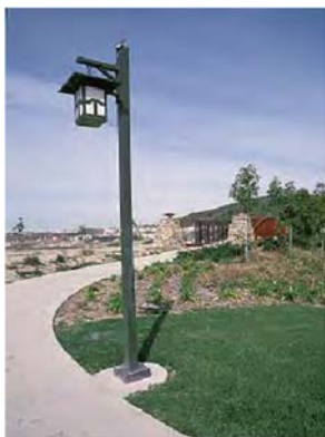
Pole-mounted site lighting fixture
