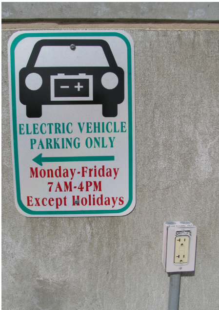
Electric vehicle parking at a City of Sacramento parking garage.
