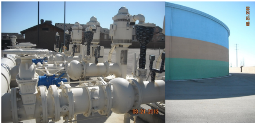
Photograph G. Pumps at the Elkhorn Tank and Pump Station Facility.
