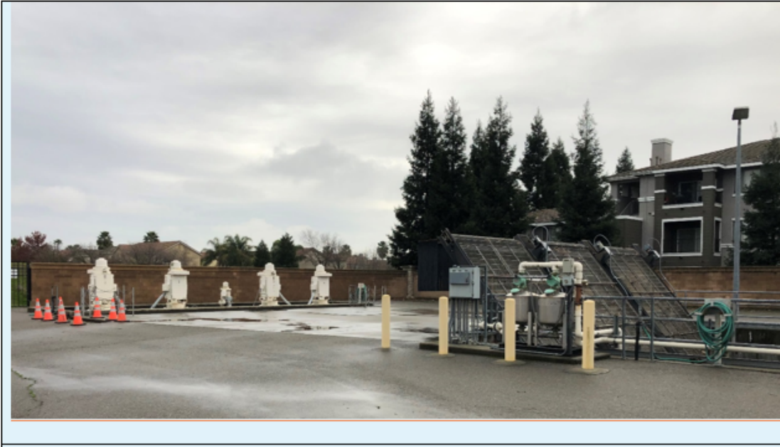
Photograph F. The pump station for Basin 11 has five pumps and a trash screen with a combined capacity of 281 cfs.
