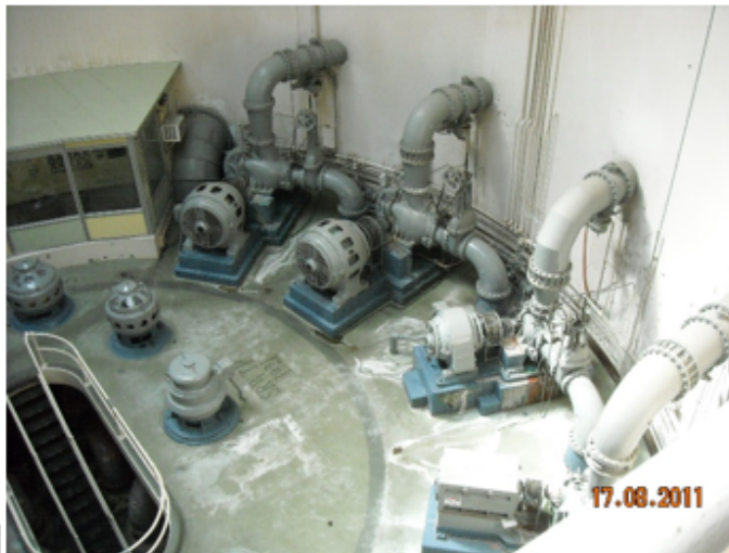
Photograph F. Sacramento River Water Treatment Plant finished water pump station.
