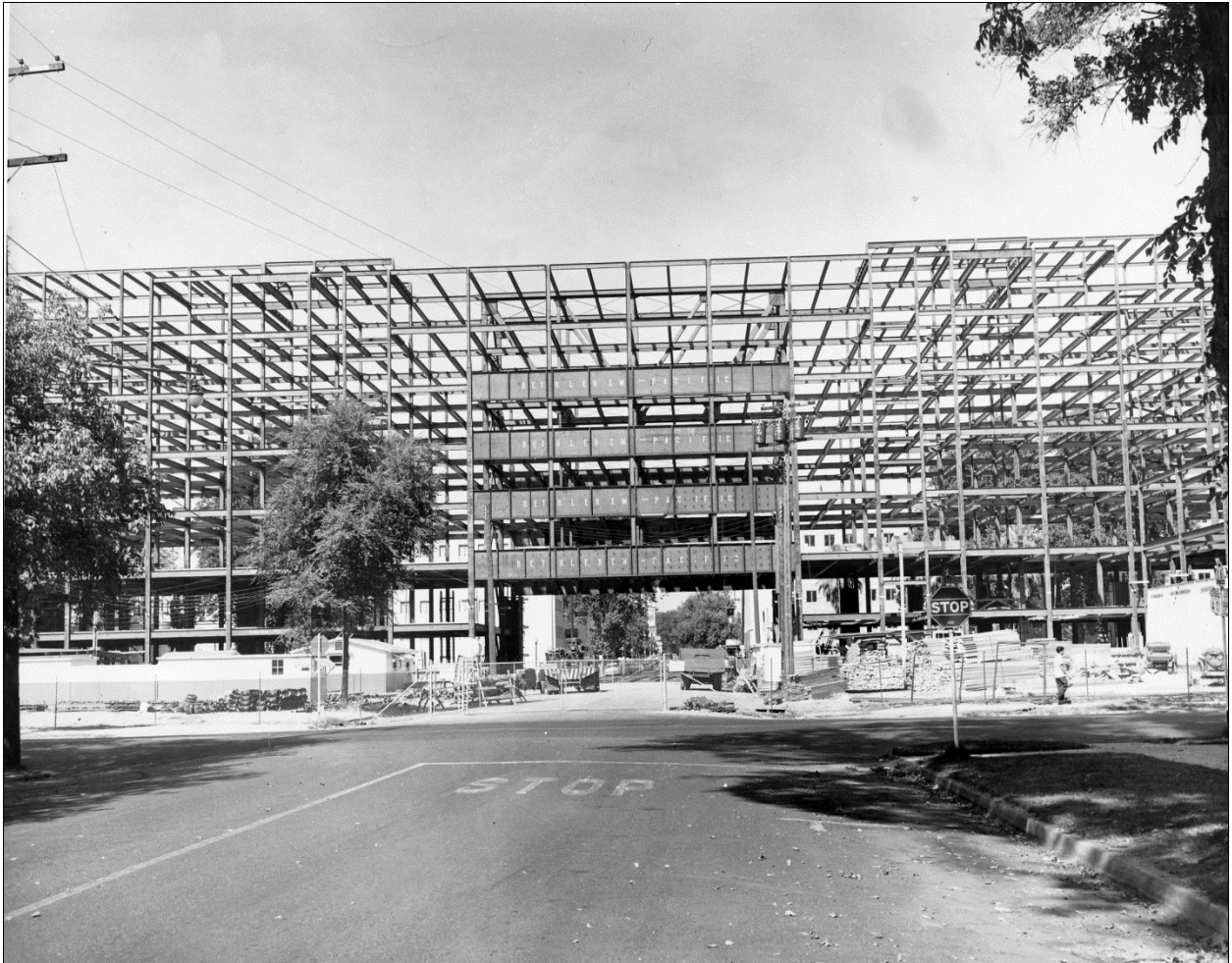
Figure 19. Construction of the Employment Development Department (EDD) Building on September 26, 1954. The building is an example of modifications made to Sacramento's original street grid to accommodate new, larger developments. [Center for Sacramento History, Ralph Shaw Collection, 1972/212/1578].
