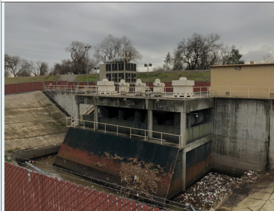
Photograph E. Pump Station 152 is located along the American River. It has five large pumps with a combined capacity of 548 cubic feet per second (cfs). The screen protects the pumps from damage from trash and debris.
