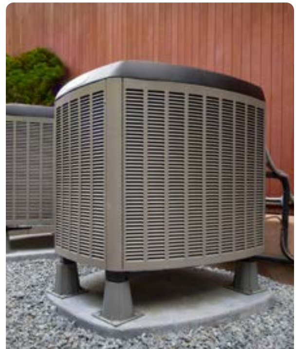
Heat Pump HVAC
