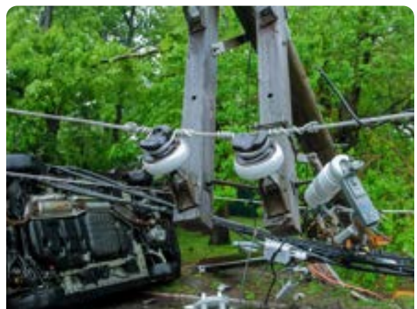
Fallen Power Pole
