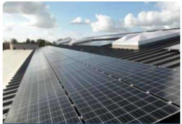
Rooftop Solar Panels
