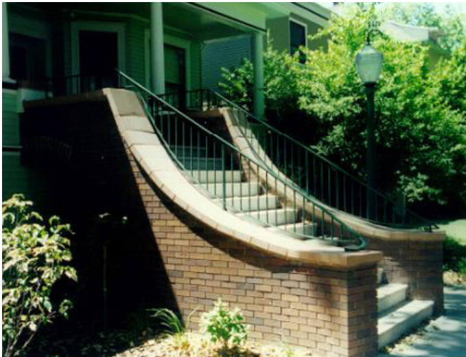
Figure 3-55. 2220 L Street. Quality Design and Detailing provide long term value for property owners and the community.
