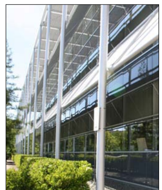
Figure 2. Applied sunshading elements on a building at Stanford University, Palo Alto, CA.
