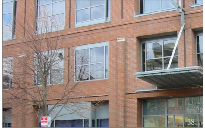
Figure 1. This building also combines curtain wall window systems with solid punched-opening walls. The wall is given a visual thickness by the varying placement of the glass line.
