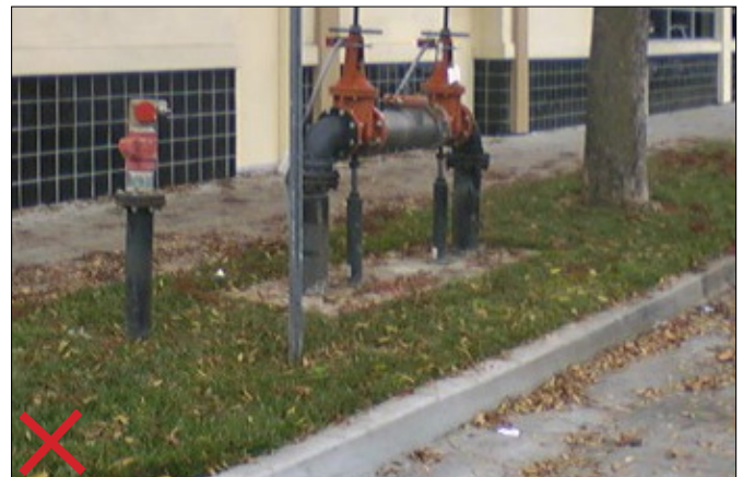
Figure 3: Utilities connections should NOT be left floating and exposed in a sidewalk's park strip.
