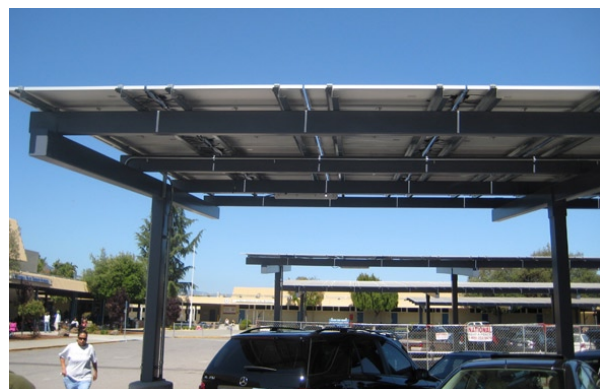
Figure 3. Canopies of photo-voltaic panel arrays covering the parking areas.
