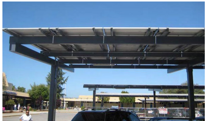
Figure 4-249. Canopies of photo-voltaic panel arrays covering the parking areas.
