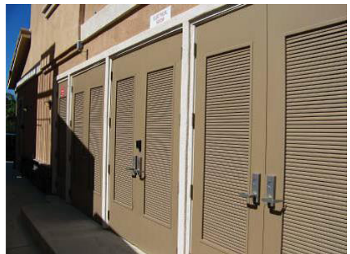
Figure 4-27. Mechanical equipment attractively screened at the rear of the building and vented to Alley.
