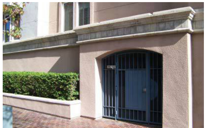
Figure 4-30. Decorative enclosure built into building façade can screen transformers and other utilities in a decorative manner.
