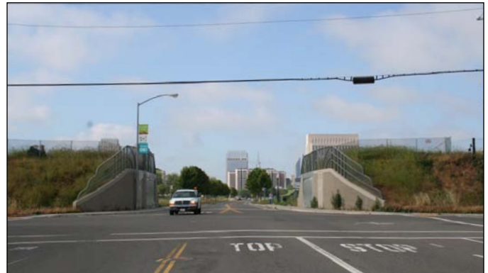
Figure 3.41. The secondary levee as seen from North 7th Street with flood gates installed in the embankment. This levee infrastructure is planned for future replacement with new grading in the Railyards plan area. With the removal of the levee that encroaches into North B Street, multiple north-south streets will connect the Railyards to the River District.
