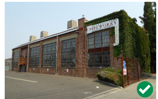
Figure 224. Steel frame windows have been preserved and maintained in this adaptively re-used building.
