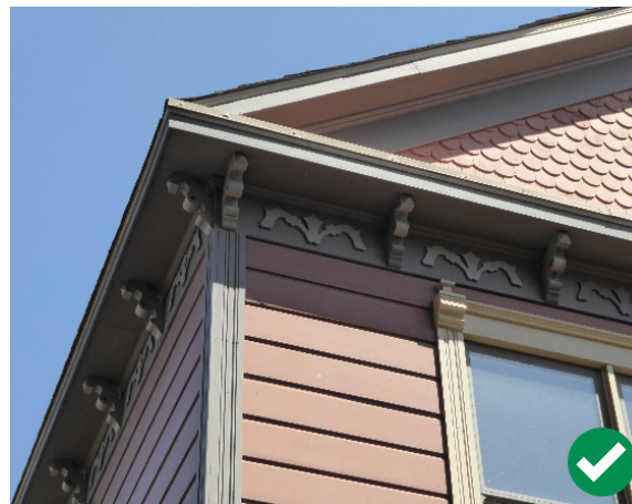
Figure 158. Many of the contributing houses in the historic district feature decorative exterior woodwork that should be maintained and preserved.
