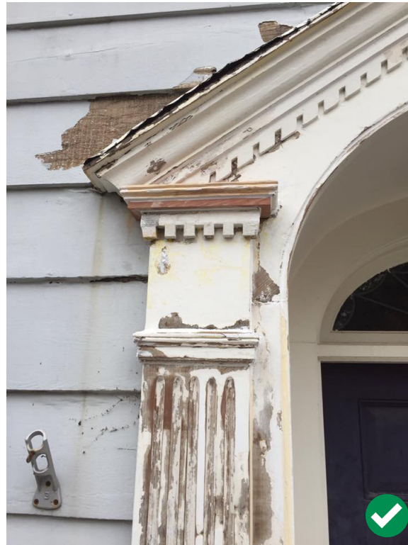
Figure 11. A new pilaster cap replaced with new wood to match the historic, damaged feature.
