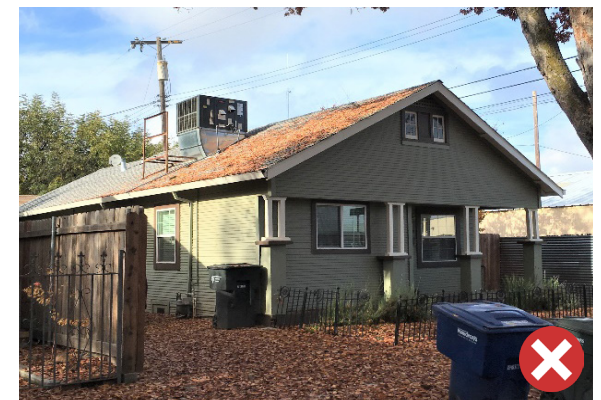
Figure 16. An example of roof-mounted mechanical equipment that is highly visible from the street.
