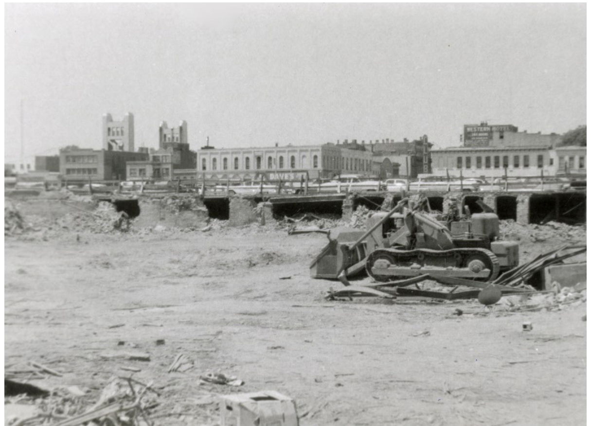
Figure 8. A demolished area of the West End as a result of the Capitol Mall and West End redevelopment project (1960). Source: Center for Sacramento History, Frank Christy Collection, 1998/722/1480.
