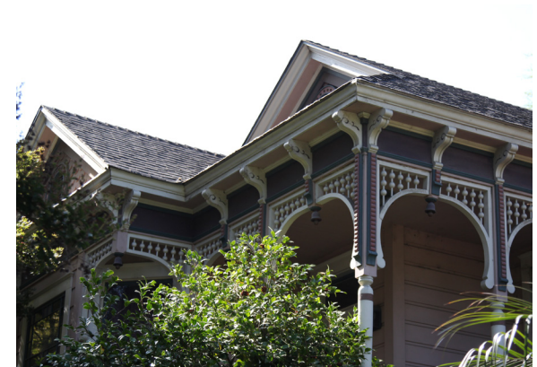
Figure 28. Decorative woodwork on a house in the Alkali Flat West Historic District.
