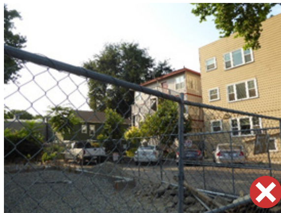
Figure 53. The use of chain link fences is prohibited.
