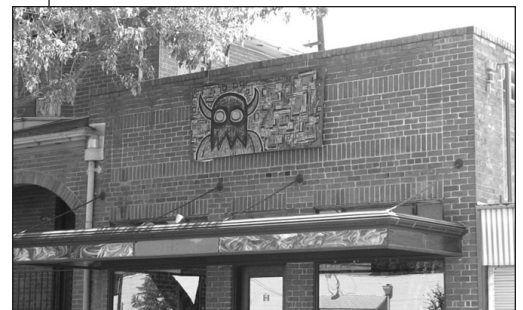
The Brick House in the Broadway Commercial Character Area has a typical flat commercial roof.
