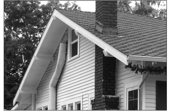
Deep eaves and overhangs can help to shade and protect the home.
