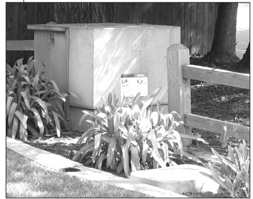
This utility box should be screened by landscaping.
