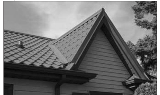
“Cool roof” options can achieve higher energy efficiency.
