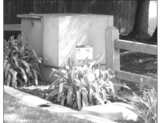
This utility box should be screened by taller growing plants.
