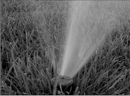
Irrigation spray head
