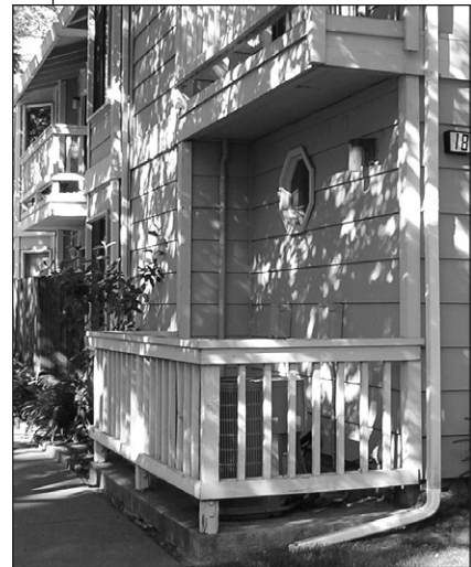
Appropriate screening of HVAC unit behind fence
