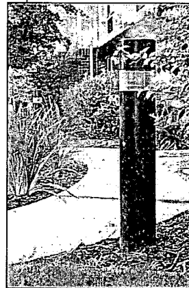
Pedestrian-scaled pathway bollard lighting
