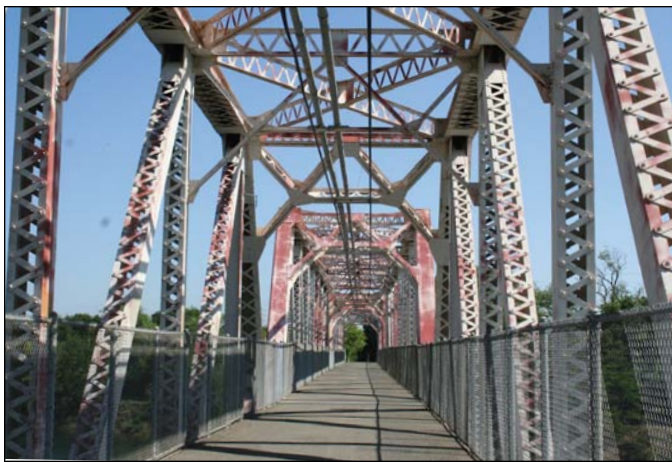
Figure 2.107. The bridge of the former Sacramento Northern Railroad once carried electrified passenger and freight service as far north as Chico, spans the river on the border of the RDSP, and is now a pedestrian-bike bridge.
