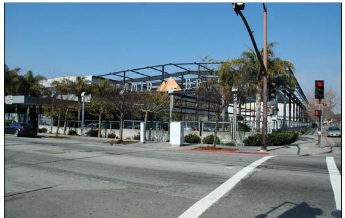
Figure 2.94. The deconstruction of a former steel-framed warehouse serves as a parking lot for the renovated masonry building housing the primary use.
