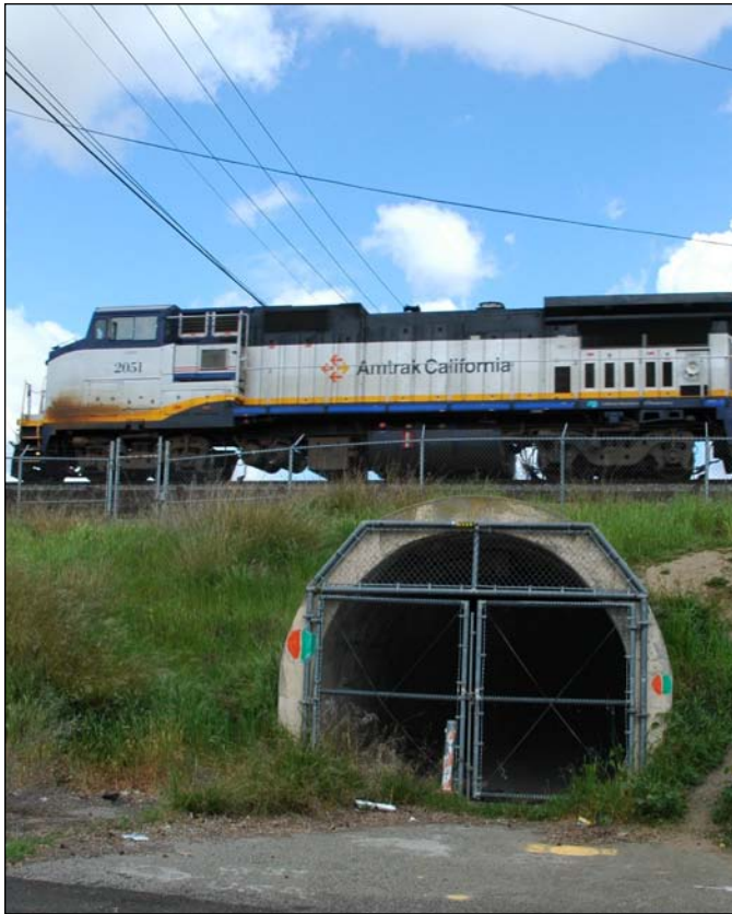
Figure 2.21. The 14th Street tunnel was closed soon after opening. When sufficient development occurs around this crossing, significant re-design will be needed to ensure better security and usability for pedestrians and cyclists.
