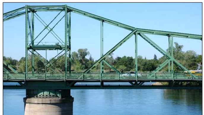
Figure 2.61. Jibboom Street Bridge is a gateway to boaters and currently the only bike connector to Discovery Park and Natomas at the confluence of the American and Sacramento Rivers. (Luis Alvarado Photo)
