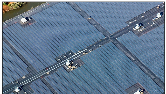
Figure 2.11. Solar photovoltaic panels cover the roof of a warehouse with accessways for roof-mounted mechanical equipment.
