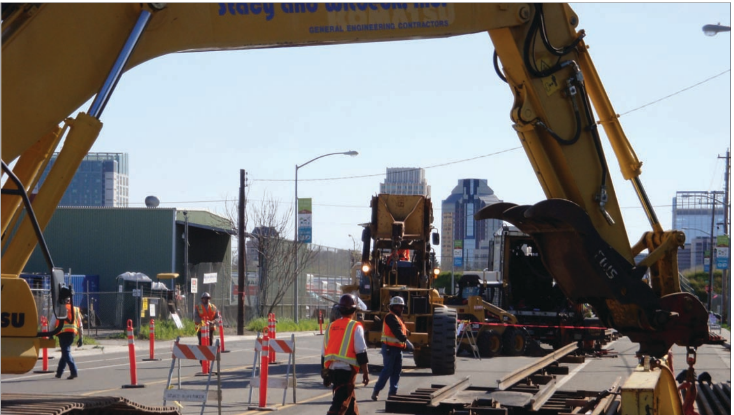
FIGURE 9.0 Light Rail Lines Being Laid on North 7th Street for the First Stop on the Green Line.
