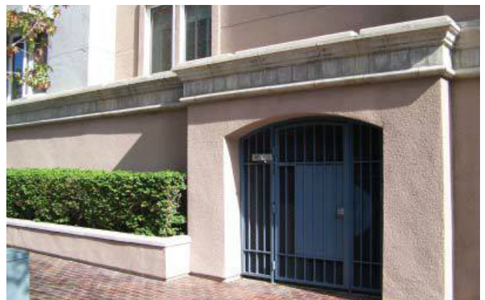
Figure 4-30. Decorative enclosure built into building façade can screen transformers and other utilities in a decorative manner.
