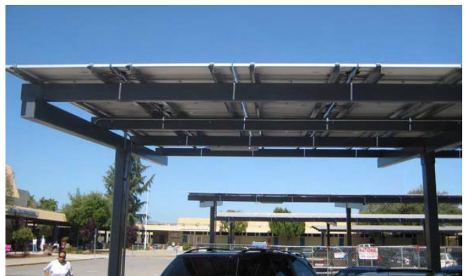
Figure 4-249. Canopies of photo-voltaic panel arrays covering the parking areas.
