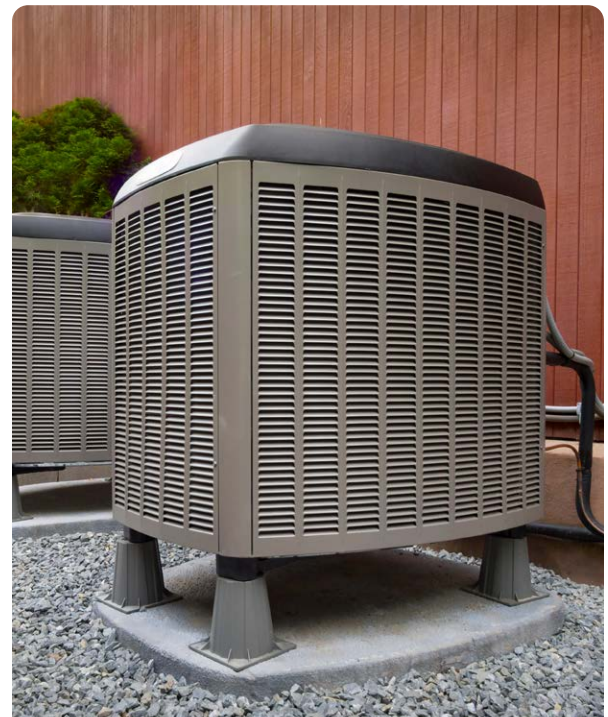
Heat Pump HVAC
