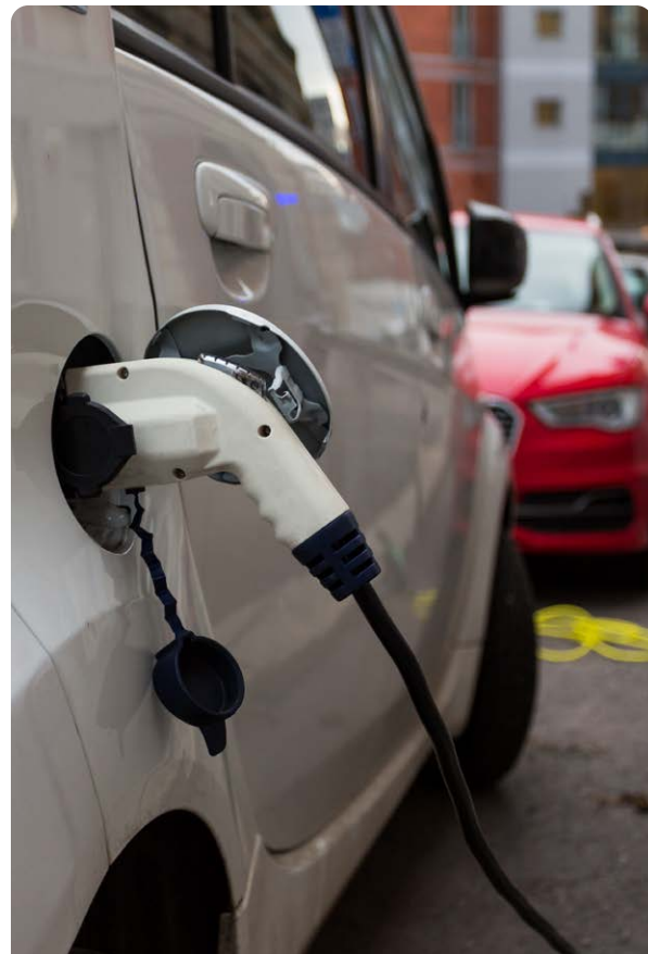
Electric Vehicle Charging
