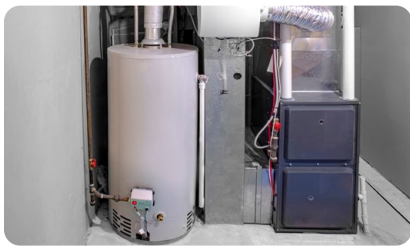
Gas Water Heater: 40-gallon storage tank
