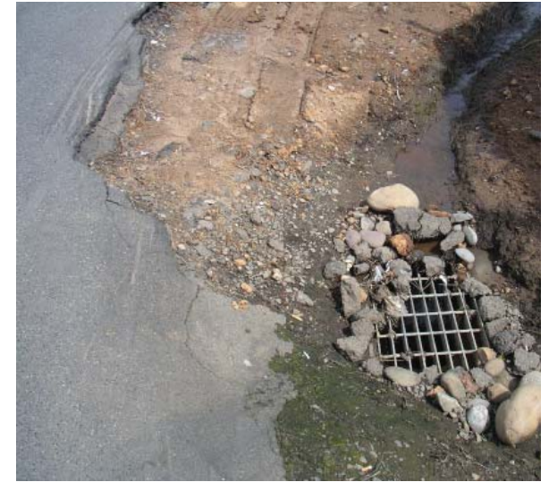
Significant drainage problems in the Dixianne neighborhood
