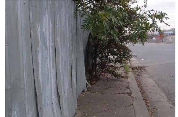
Poor pedestrian connections
