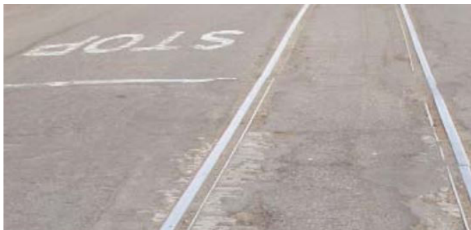
Figure 6-155. Abandoned rail tracks on contribute to varying pavement conditions.
