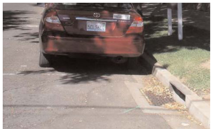
Figure 6-141. Existing curbs and gutters should be maintained in the short term.
