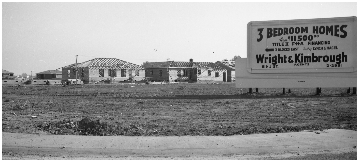
FHA financed homes under construction in Land Park. The advertised use of Title II FHA loans during this period indicates the use of racial restrictions on non-White residency. Circa 1942. Source: Center for Sacramento History
