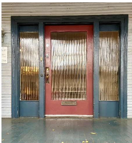
FIGURE 9: THE FLUTED GLASS FRONT DOOR AND SIDELIGHTS ARE CHARACTER-DEFINING FEATURES OF 2224 J ST.
