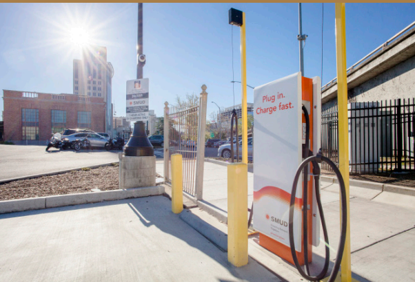
New Electric Vehicle DC Fast Charger
