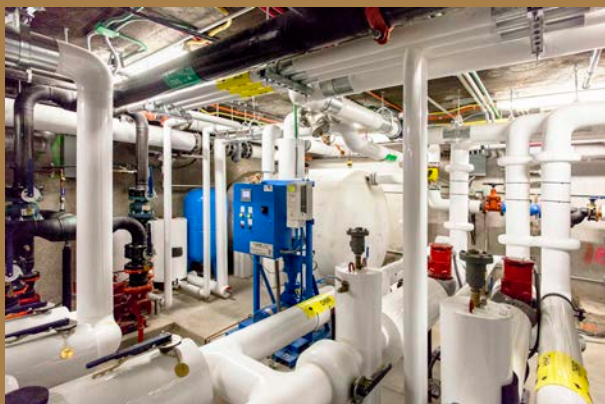
SVS High-Efficiency Mechanical System and Rain Water Catchment
