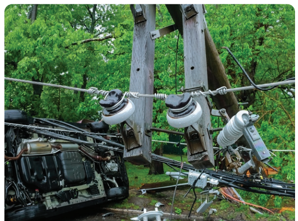
Fallen Power Pole
