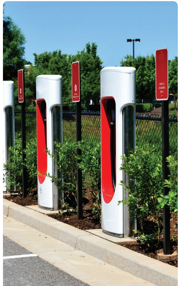
EV Charging Stations
