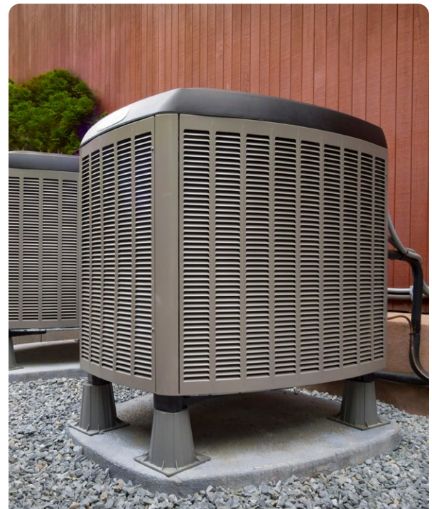
Heat Pump HVAC
