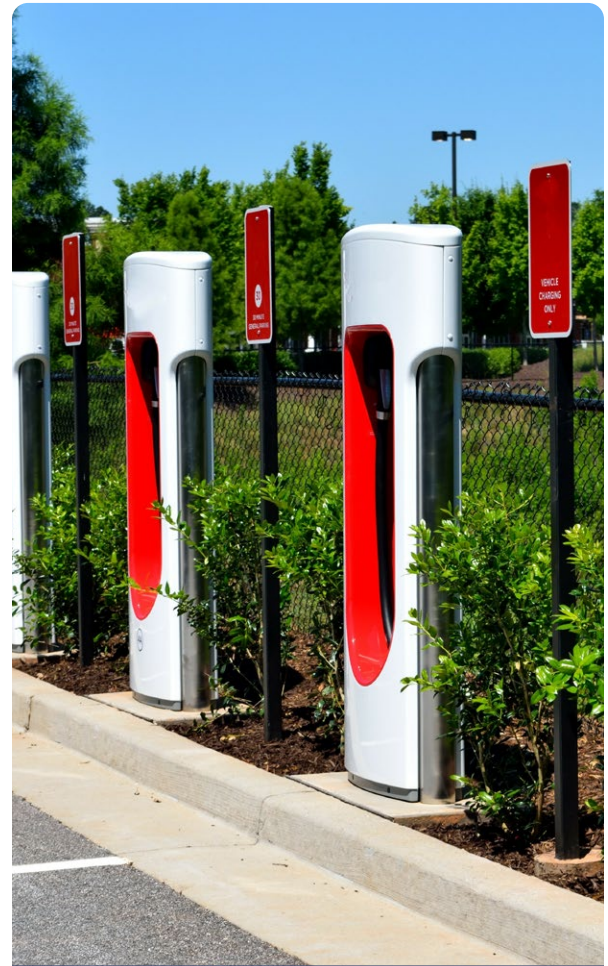
EV Charging Stations
