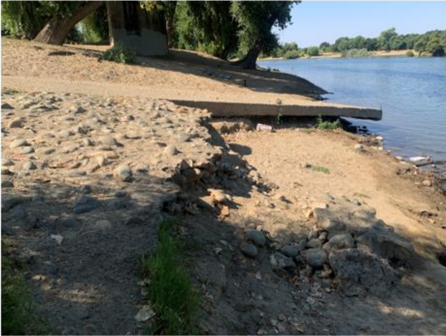
Tiscornia Boat Ramp Erosion& Undercutting at 2.6 ft high tide
