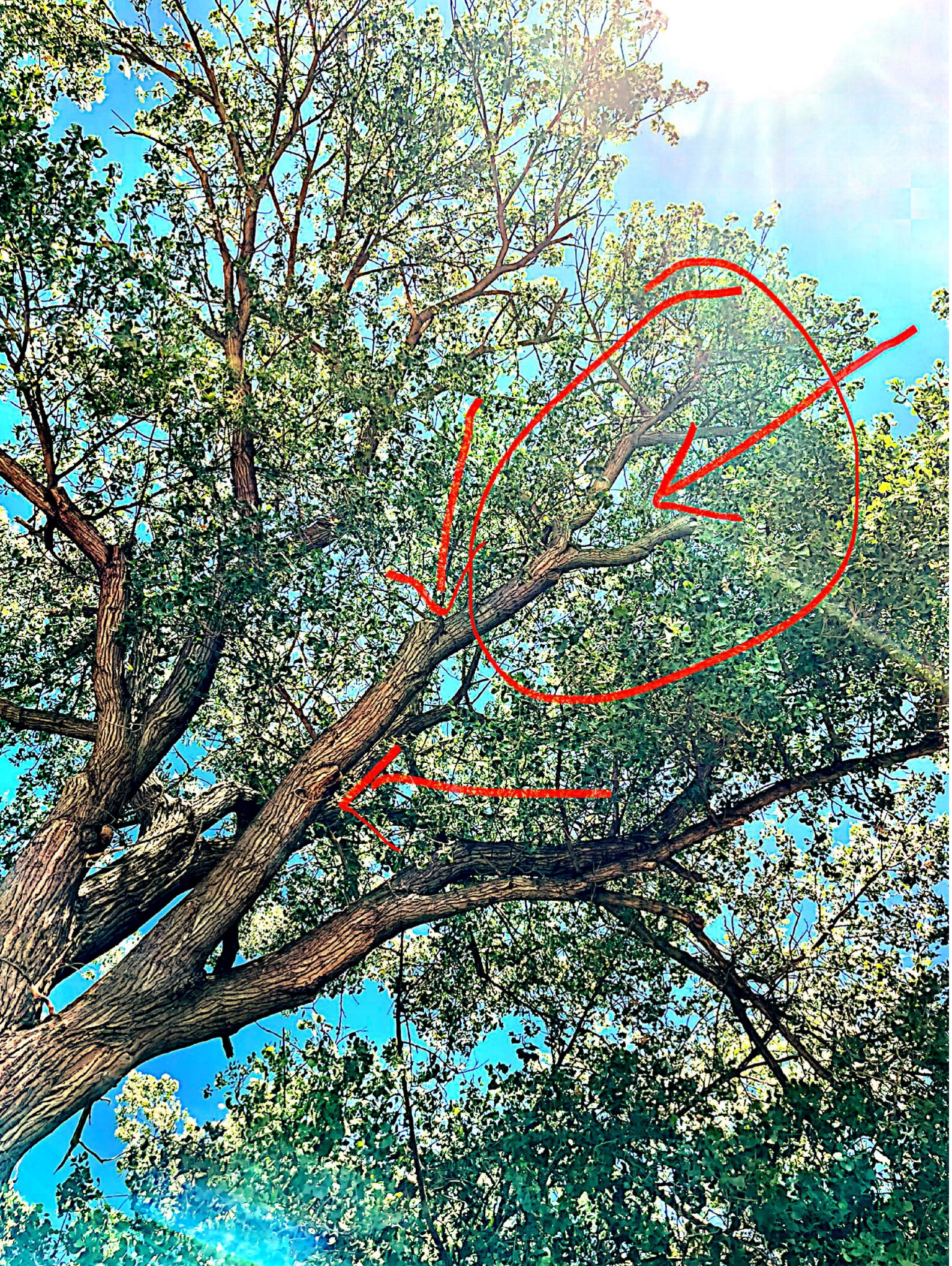
Old Failures and rams head connection
