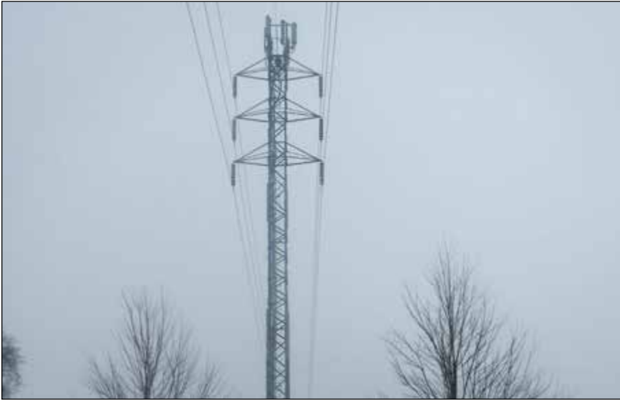
Photo 1: Transmission Line with Cell Tower Infrastructure Facing North
