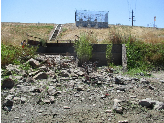
Photo 21. View looking south toward the Sump 154 concrete outfall structures from the dry bed of Arcade Creek. Some riprap occurs below the outfall. 23 July 2020.
