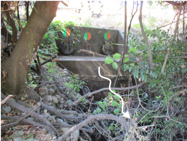
Photo 1. View looking northeast toward the Sump 58 Outfall Channel as it leaves the outfall structure and enters a heavily eroded channel. 23 July 2020.
