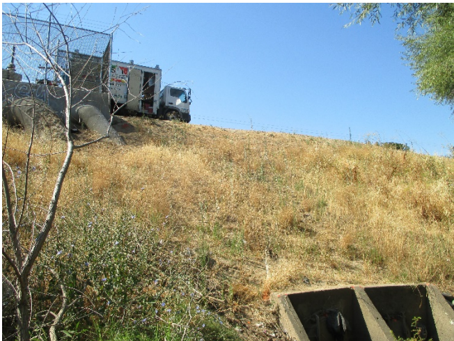
Photo 31. View looking south toward the alignment of the Sump 159 outfall pipes on the water side of the levee. Nonnative grassland occurs on the levee slope. 23 July 2020.
