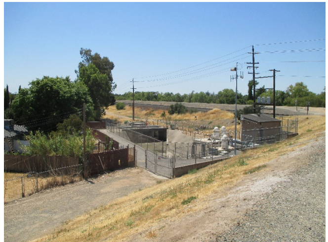
Photo 24. View looking southwest toward the fenced Sump 154 facility on the land side of the levee. 23 July 2020.
