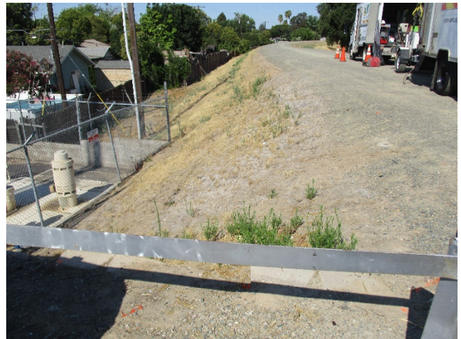
Photo 32. View looking southwest along the land side of the levee. The fenced Sump 159 facility is on left. 23 July 2020.
