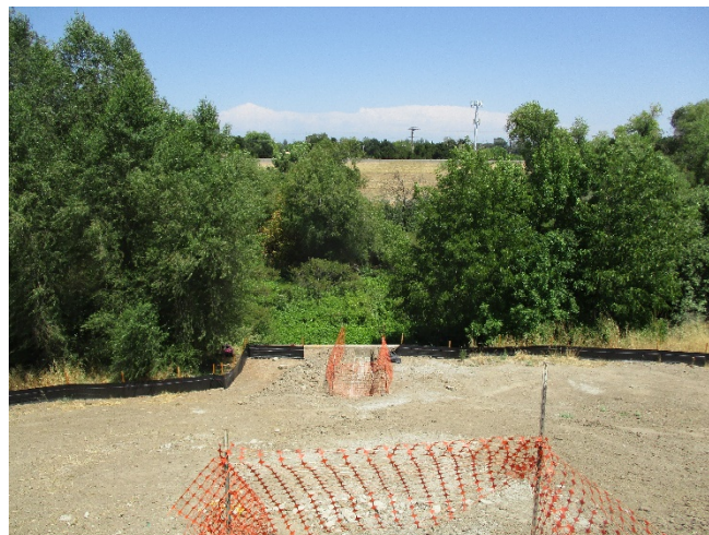
Photo 12. View looking east along the Sump 102 outfall pipe alignment from the levee crest. This area was under construction during fieldwork. 23 July 2020.
