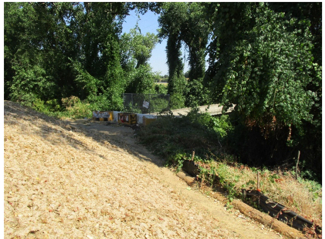
Photo 4. View looking southeast toward the upper portion of the waterside levee slope along Garden Highway. 23 July 2020.
