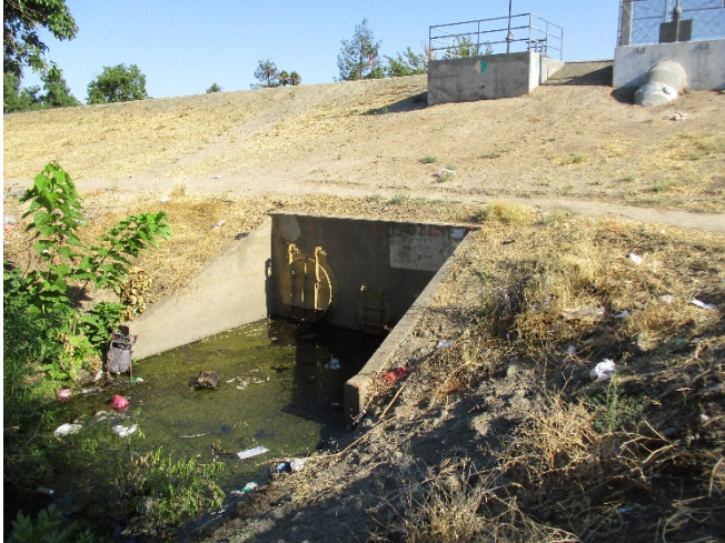
Photo 13. View looking northwest toward the Sump 103 outfall as it enters Arcade Creek. The banks around the outfall have been reinforced with concrete. 23 July 2020.
